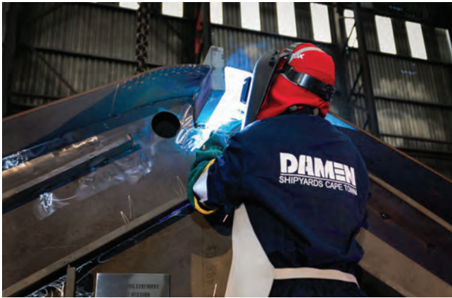
Apprentice Welder Jenny-Lee Fortuin welds the coin to the keel for the second of three multimission, inshore patrol vessels that Damen Shipyards Cape Town is building.
