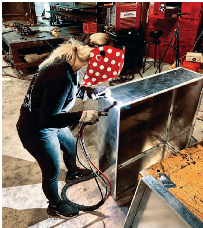
Fig. 1 — Stephanie Hoffman welds the beveled edges of the Statue of Liberty base. (Photo courtesy of Hoffman's Instagram @underground_metal_works .)
