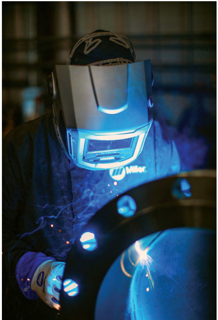
Fig. 1 — A switch to the Regulated Metal Deposition (RMD®) process eliminated back purge on stainless steel pipe welds, saving significant time and money.
